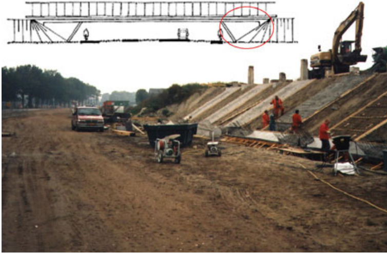
Figure 8.13: Construction of an overpass with a picture of the initial design (A30, the Netherlands). Photo by Laurens Jansen.
